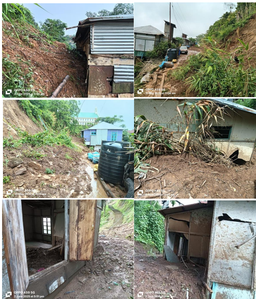
Figure 3 Houses affected by landslides
